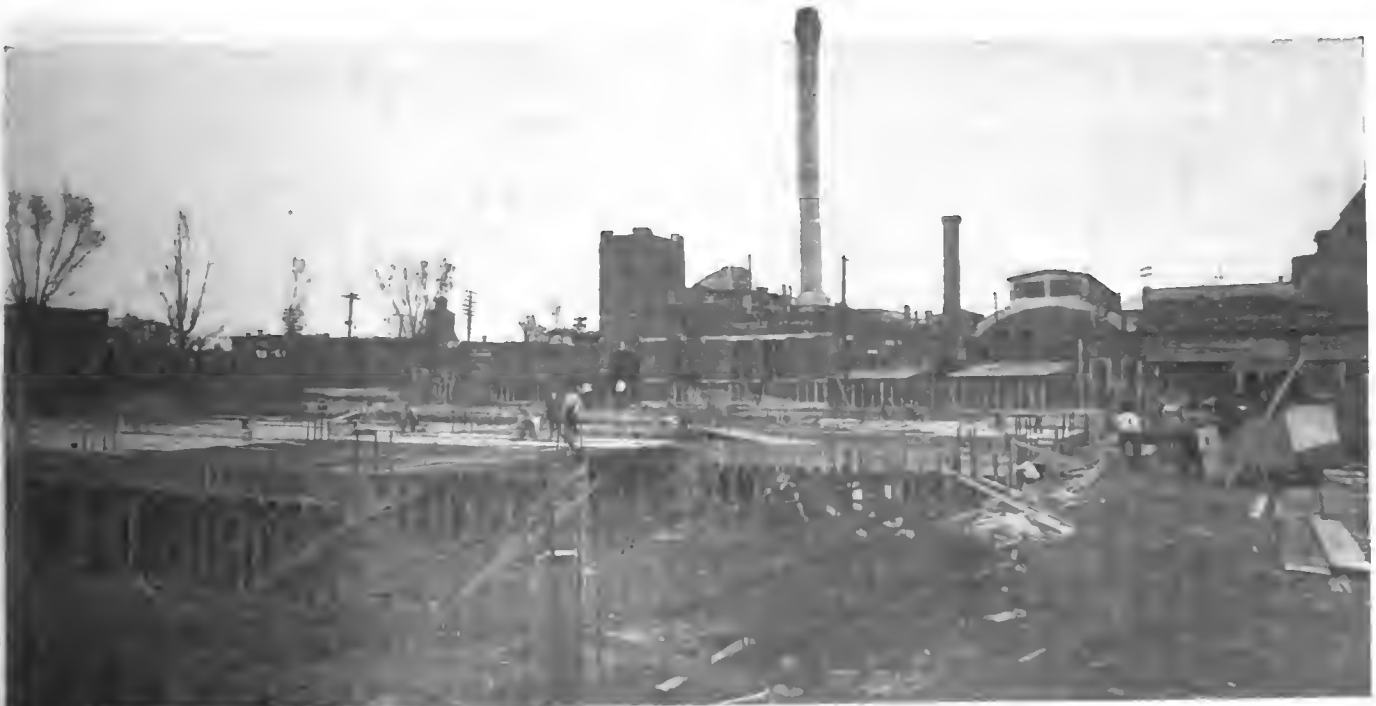
Additional floor space in their factory, to the amount of 70,000 square feet, will be gained by the erection of another big building by Wheeler & Schebler, makers of the Schebler carbureter, at Indianapolis. The building is now in course of construction. It will be three stories, of reinforced concrete and will give facilities for 200 more employees, raising the total product of the company to 1,000 carbureters a day. The company has now installed gas engines developing 350 horsepower.
